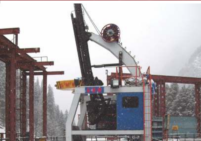
TRCM with Additional Gate/Trash Rack Lifting Mechanism
